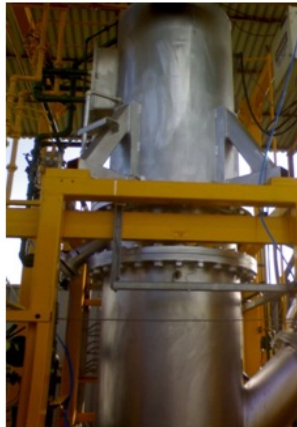
Picture 8: Secondary Combustion Chamber
