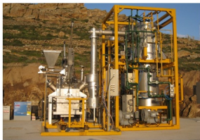
Picture 3: General view of the demonstration gasification / vitrification unit
